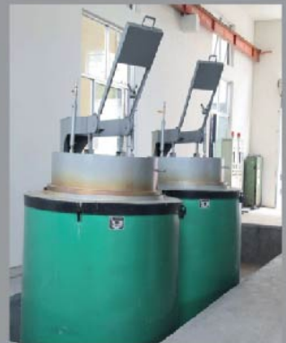
Shaft normalizing furnace
